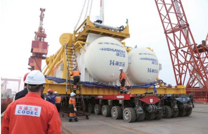
Offshore installation of the first commercial subsea data center in the world
