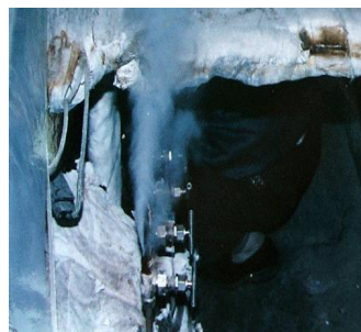
High risk of steam leakage
